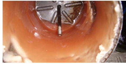
Filter Blocked Due to Wax Deposit
