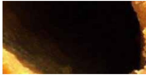
Blocked Fuel Filters and Pipes
