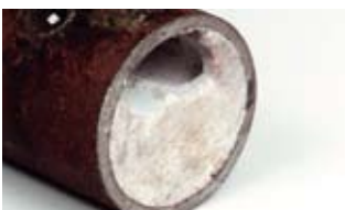
An examples of scale, resulting in severe reduction in water circulation
