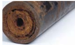
Contaminants can cause reduction in circulation, and erosion of piping, pump impellers, etc.
