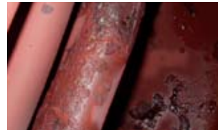
Corrosion can cause dangerous leaks
